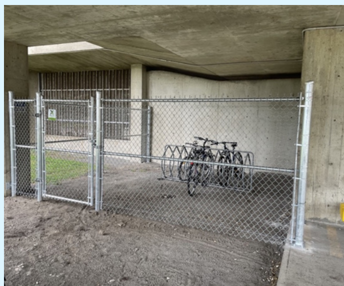
Theft-protected bike parking lot, adjacent to existing bike parking area in front of the main entrance of the Institute. Electric charging access will soon be available Source : Institut national de psychiatrie légale Philippe-Pinel
